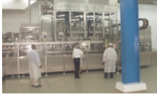
UHT milk filling at Beyti Dairy on an aseptic linear Asbofill machine
